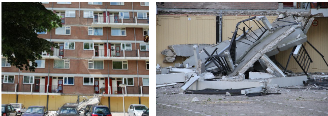
Fig. 1. Unannounced collapse of gallery plates in an apartment building in Leeuwarden, The Netherlands, 2013
